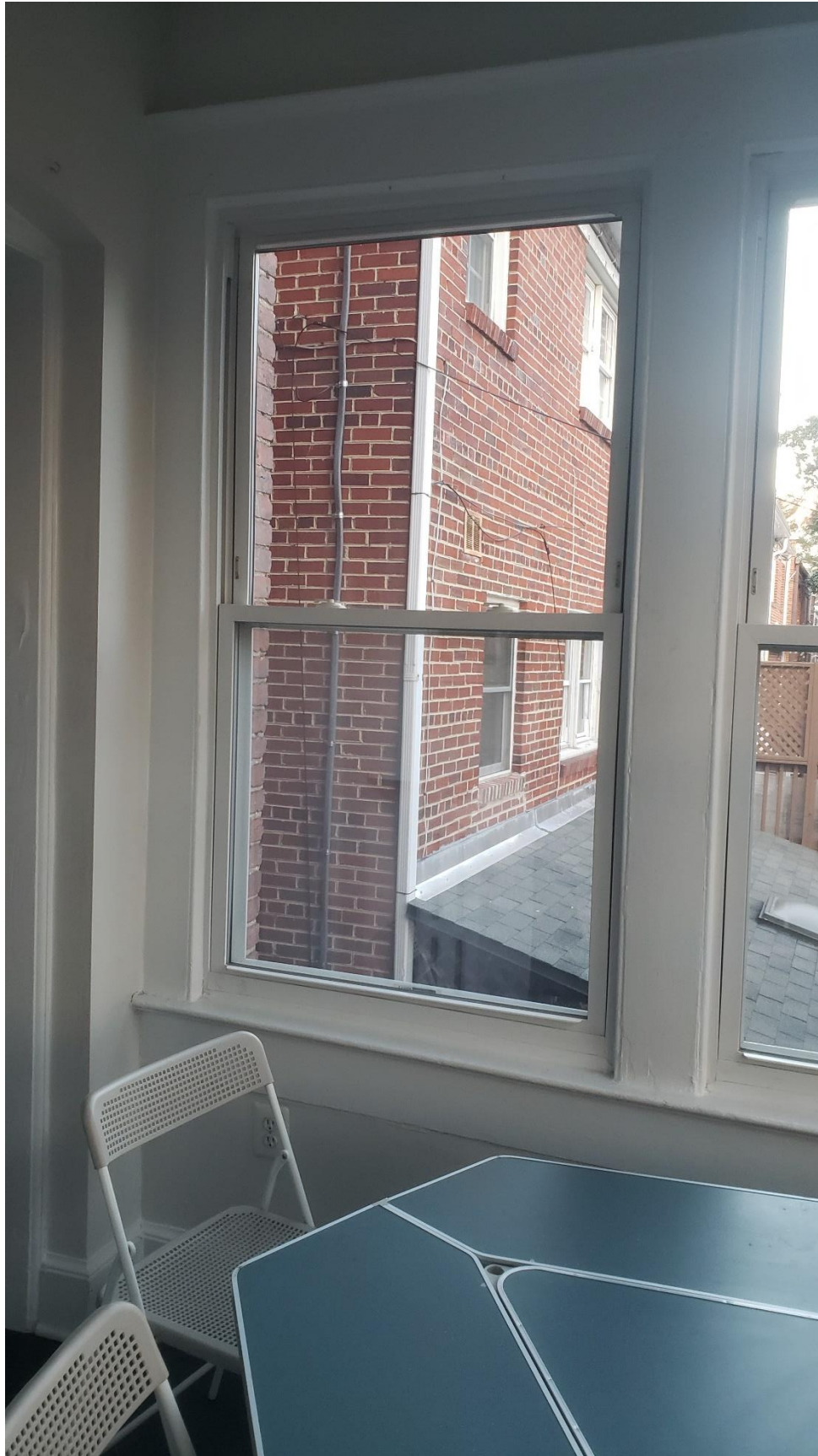
Breakfast Room, facing East. Showing alignment of current structures and distance between them
